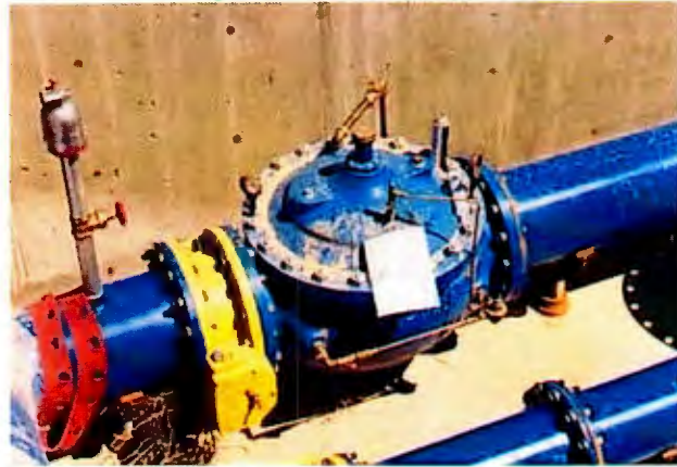
Pressure-reducing valves as energy opportunities
