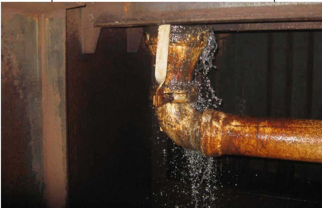
Figure 22. Photo. Clogged drain leaking water onto superstructure.
