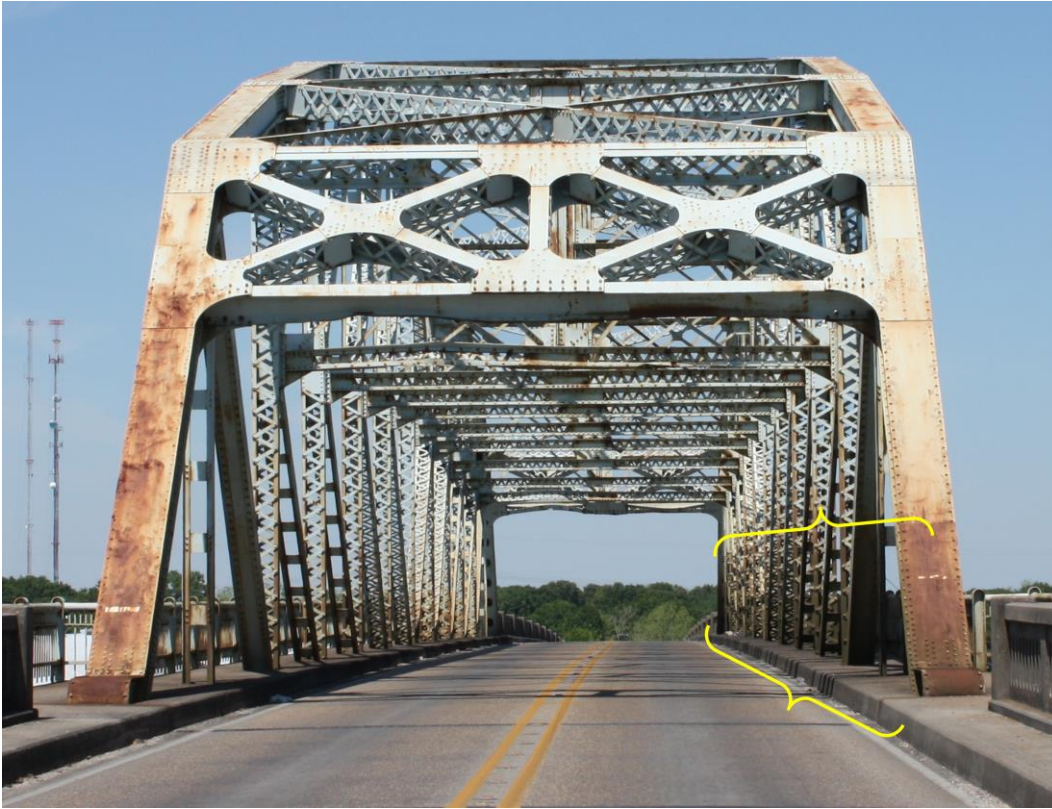
Figure 23. Photo. Through truss showing darkened area in close proximity to the travel lane (i.e. splash zone) that is corroding faster than other parts of the truss outside the splash zone.
