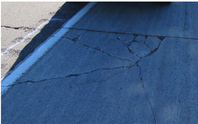
Figure 3. Corner-cracked panel adjoining thermally cracked asphalt shoulder in 5-inch (125 mm) unbonded overlay
