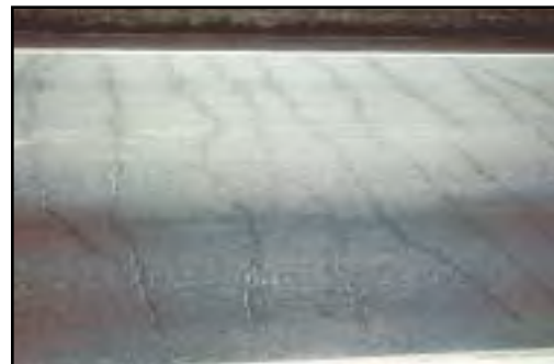
FIGURE 97 Distress Type CRCP 3—Transverse Cracking Pattern
