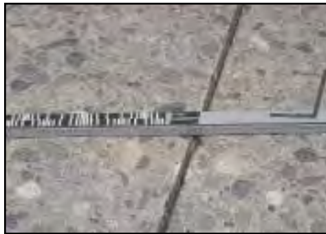
FIGURE 133 Distress Type CRCP 15—Longitudinal Joint Seal Damage
