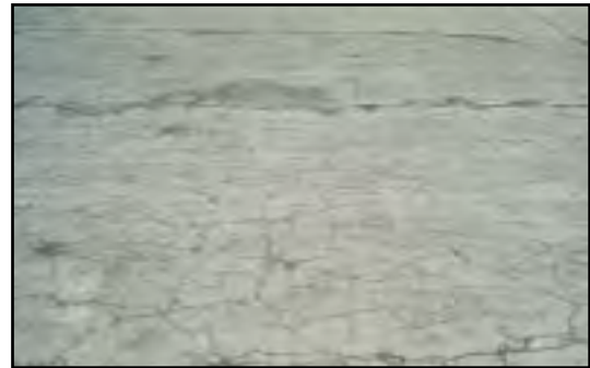
FIGURE 69 Distress Type JCP 8a—Map Cracking
