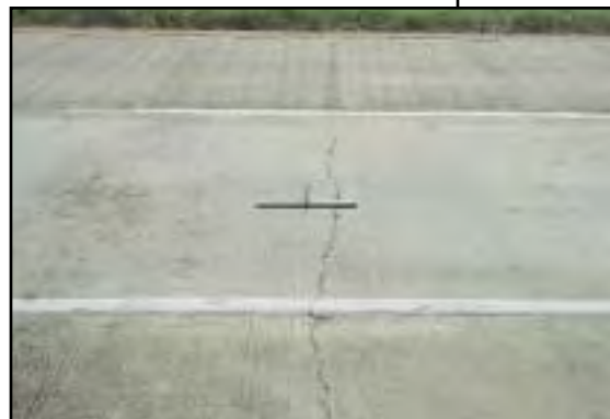
FIGURE 99 Distress Type CRCP 3—Moderate Severity Transverse Cracking
