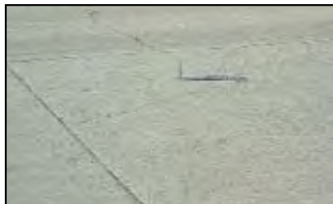
FIGURE 49 Distress Type JCP 1—Low Severity Corner Break
