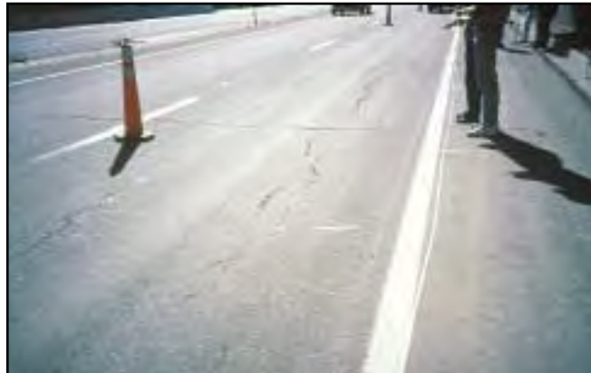
FIGURE 5 Distress Type ACP 1—Low Severity Fatigue Cracking
