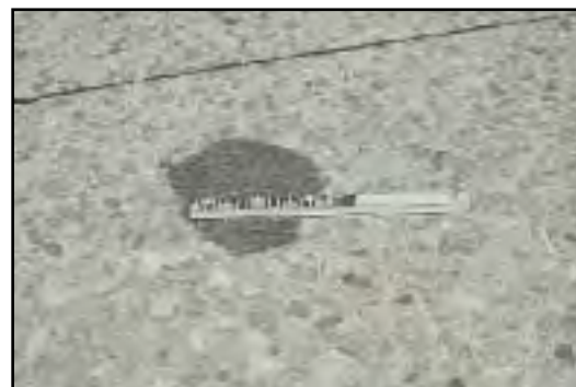
FIGURE 85 Distress Type JCP 15—Small, Low Severity Asphalt Concrete Patch
