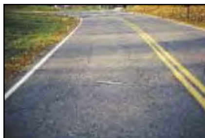
FIGURE 9 Distress Type ACP 2—Block Cracking with Fatigue Cracking in the Wheel Paths
