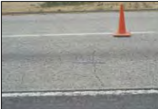
FIGURE 98 Distress Type CRCP 3—Low Severity Transverse Cracking
