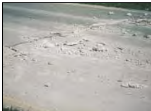
FIGURE 107 Distress Type CRCP 7—A Blowup
