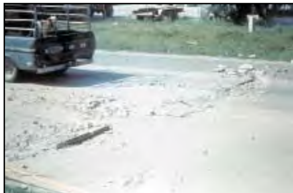
FIGURE 76 Distress Type JCP 11—A Blowup
