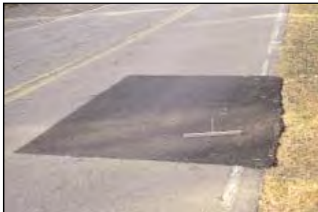
FIGURE 24 Distress Type ACP 7—Moderate Severity Patch
