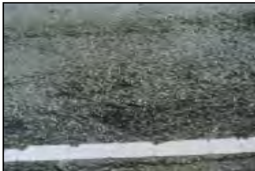
FIGURE 41 Distress Type ACP 13—Loss of Fine and Some Coarse Aggregate
