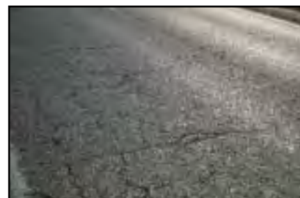
FIGURE 10 Distress Type ACP 2—High Severity Block Cracking
