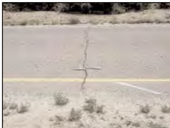
FIGURE 21 Distress Type ACP 6—High Severity Transverse Cracking
