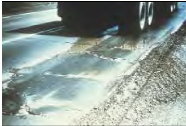
FIGURE 89 Distress Type JCP 16—Water Bleeding and Pumping
