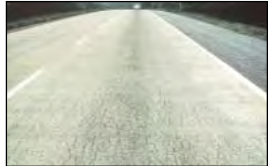
FIGURE 101 Distress Type CRCP 4a—Map Cracking Attributable to Alkali-Silica Reactivity
