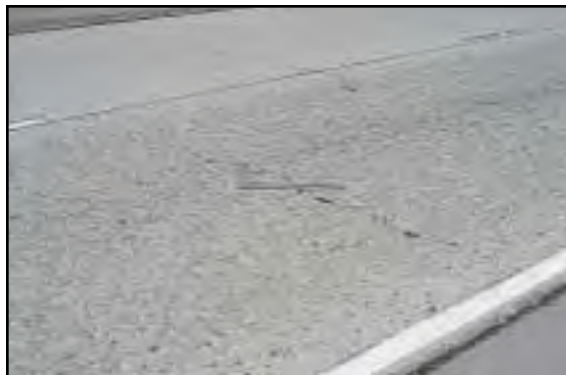
FIGURE 60 Distress Type JCP 4—High Severity Transverse Cracking
