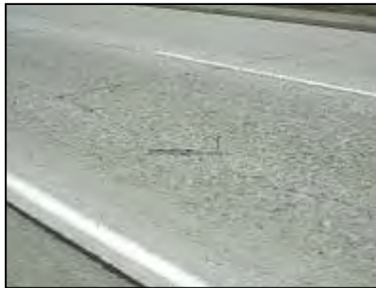
FIGURE 56 Distress Type JCP 3—Moderate Severity Longitudinal Cracking
