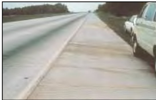
FIGURE 131 Distress Type CRCP 14—Water Bleeding and Pumping
