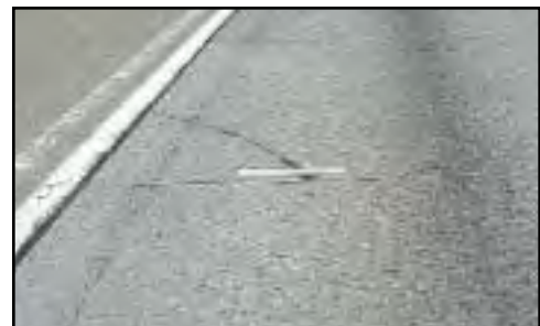
FIGURE 50 Distress Type JCP 1—Moderate Severity Corner Break
