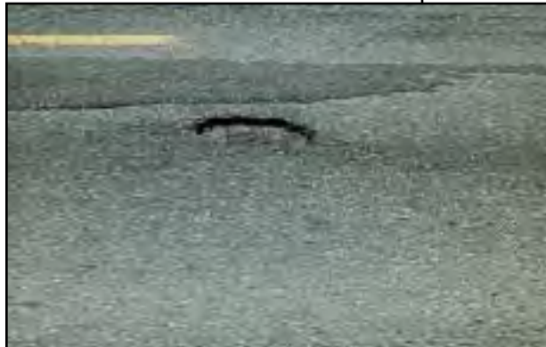
FIGURE 28 Distress Type ACP 8—Moderate Severity Pothole
