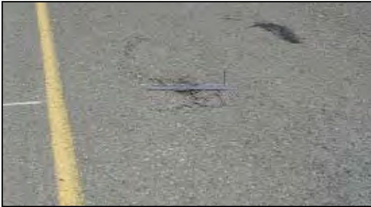
FIGURE 27 Distress Type ACP 8—Low Severity Pothole
