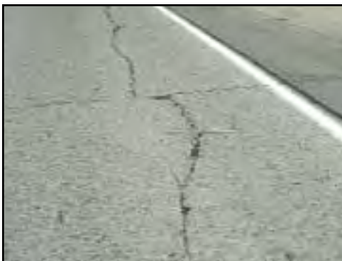
FIGURE 57 Distress Type JCP 3—High Severity Longitudinal Cracking
