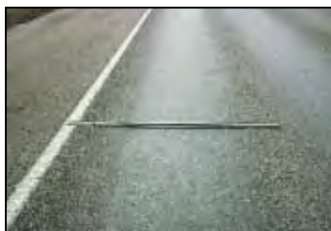
FIGURE 32 Distress Type ACP 9—Rutting
