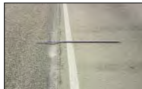
FIGURE 115 Distress Type CRCP 9—Lane-to-Shoulder Dropoff
