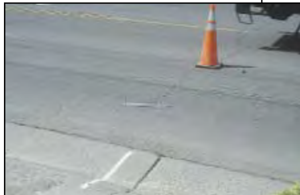
FIGURE 20 Distress Type ACP 6—Moderate Severity Transverse Cracking
