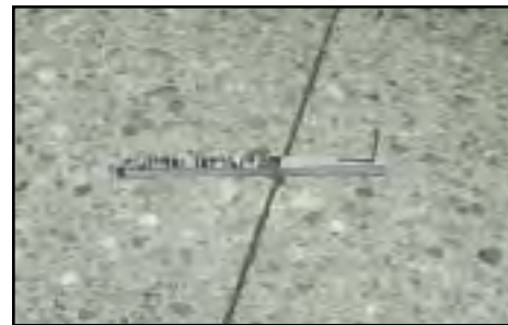
FIGURE 61 Distress Type JCP 5—Low Severity Joint Seal Damage
