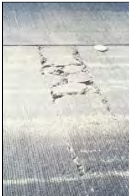
FIGURE 126 Distress Type CRCP 12—High Severity Punchout
