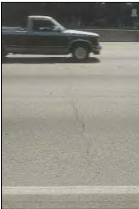
FIGURE 19 Distress Type ACP 6—Low Severity Transverse Cracking
