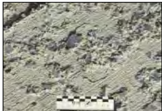
FIGURE 71 Distress Type JCP 8b—Scaling, Close-up View
