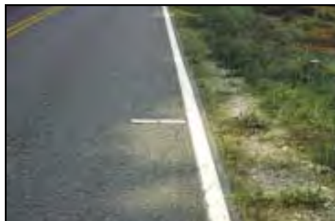
FIGURE 12 Distress Type ACP 3—Low Severity Edge Cracking
