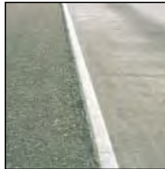
FIGURE 83 Distress Type JCP 14—Well-Sealed Lane-to-Shoulder Separation
