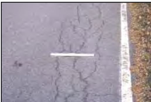
FIGURE 6 Distress Type ACP 1—Moderate Severity Fatigue Cracking
