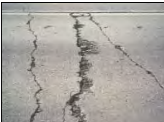
FIGURE 100 Distress Type CRCP 3—High Severity Transverse Cracking
