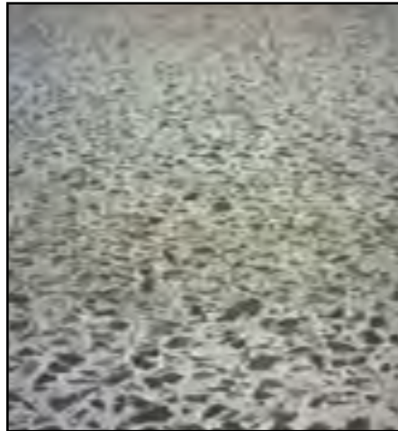
FIGURE 103 Distress Type CRCP 5—Polished Aggregate
