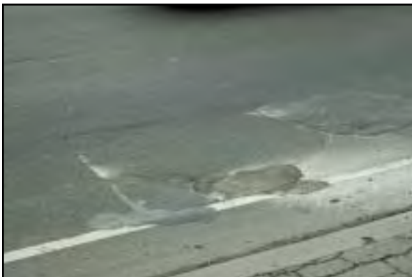
FIGURE 25 Distress Type ACP 7—High Severity Patch
