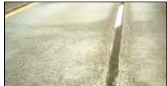
FIGURE 92 Distress Type CRCP 1—High Severity “D” Cracking at Longitudinal Joint
