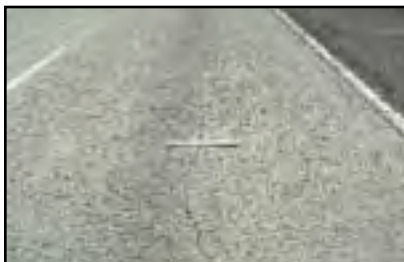
Figure 94 Distress Type CRCP 2—Low Severity Longitudinal Cracking
