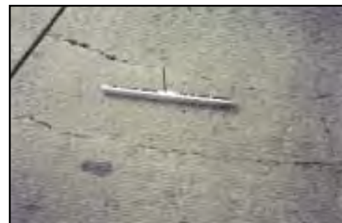
FIGURE 124 Distress Type CRCP 12—Low Severity Punchout
