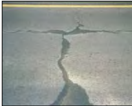
FIGURE 45 Distress Type ACP 15—Water Bleeding and Pumping
