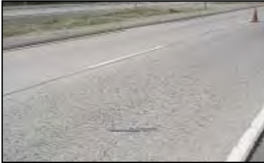
FIGURE 55 Distress Type JCP 3—Low Severity Longitudinal Cracking
