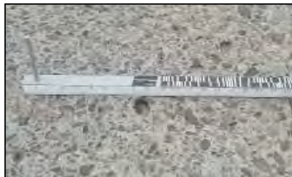
FIGURE 105 Distress Type CRCP 6—Popouts
