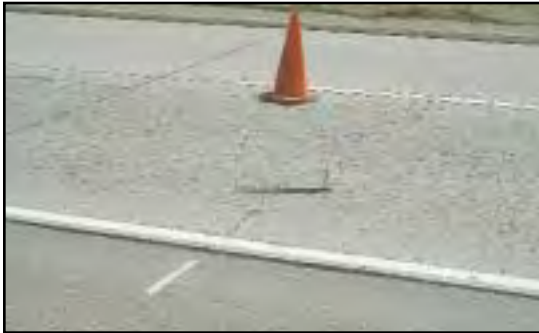
FIGURE 59 Distress Type JCP 4—Moderate Severity Transverse Cracking
