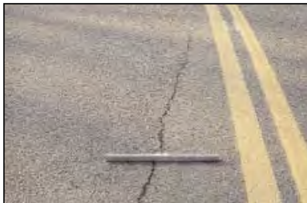
FIGURE 15 Distress Type ACP 4b—High Severity Longitudinal Cracking not in the Wheel Path
