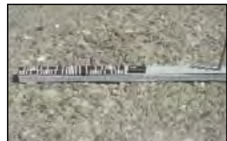
FIGURE 42 Distress Type ACP 13—Loss of Coarse Aggregate
