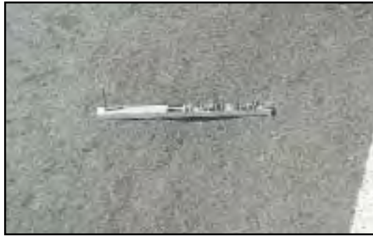
FIGURE 40 Distress Type ACP 13—Loss of Fine Aggregate
