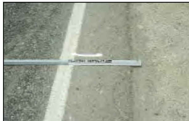
FIGURE 44 Distress Type ACP 14—Lane-to-Shoulder Dropoff
