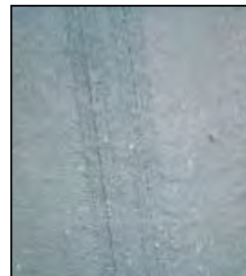
FIGURE 38 Distress Type ACP 11— Aggregate Obscured
