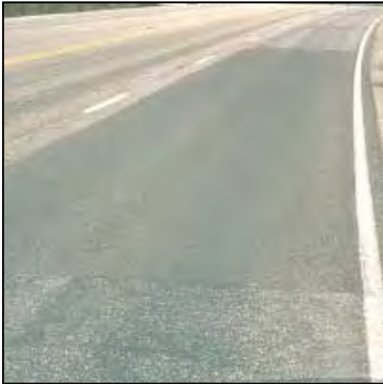
FIGURE 23 Distress Type ACP 7—Low Severity Patch
