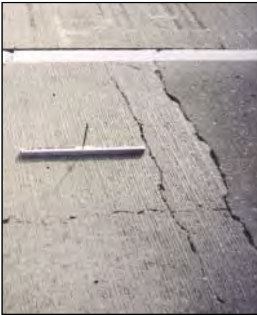
FIGURE 125 Distress Type CRCP 12—Moderate Severity Punchout
