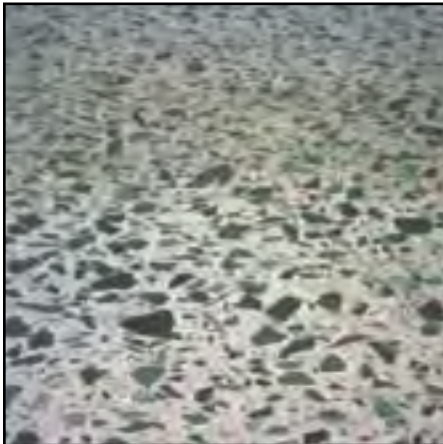
FIGURE 72 Distress Type JCP 9—Polished Aggregate
