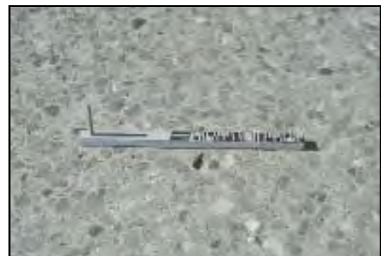
FIGURE 74 Distress Type JCP 10—A Popout
