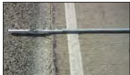
FIGURE 80 Distress Type JCP 13— Lane-to-Shoulder Dropoff
