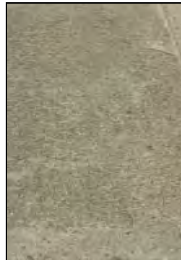
FIGURE 102 Distress Type CRCP 4b—Scaling
