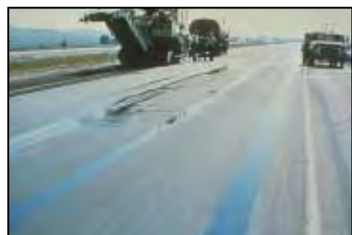
FIGURE 33 Distress Type ACP 9—Standing Water in Ruts
