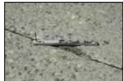
FIGURE 68 Distress Type JCP 7—Moderate Severity Spalling of Transverse Joint, Close-up View
