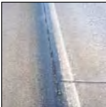
FIGURE 82 Distress Type JCP 14—Poorly Sealed Lane-to-Shoulder Separation
