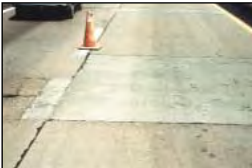
FIGURE 122 Distress Type CRCP 11—Low Severity Portland Cement Concrete Patch
