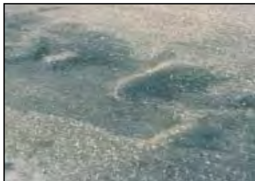
FIGURE 35 Distress Type ACP 10—Shoving in Pavement Surface
