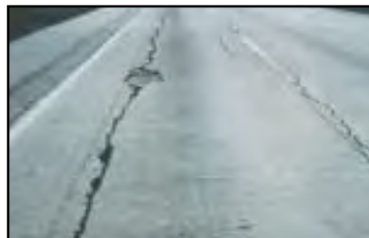
FIGURE 95 Distress Type CRCP 2—High Severity Longitudinal Cracking
