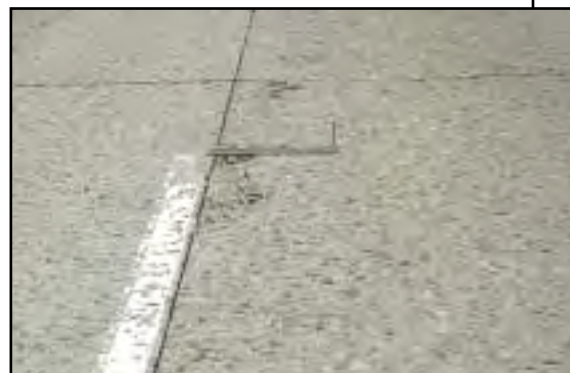
FIGURE 65 Distress Type JCP 6—High Severity Spalling of Longitudinal Joint
