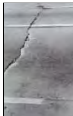
FIGURE 78 Distress Type JCP 12—Faulting of Transverse Cracks
